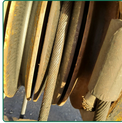
Head Sheaves and bearings
